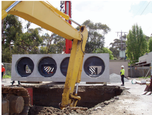
Overflow Storage Tank
